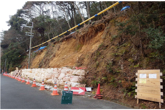
Right after slope failure
