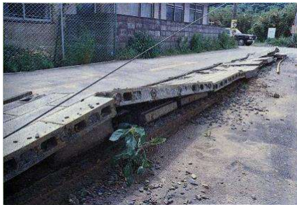
Crashed concrete block wall
